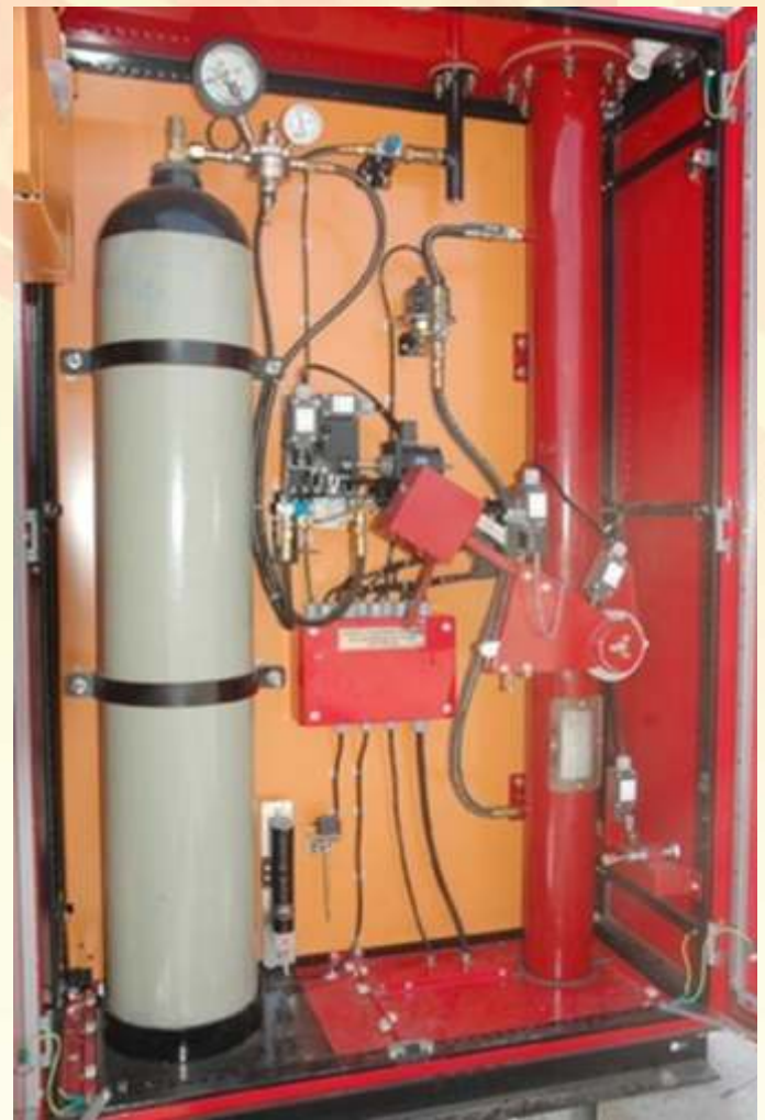
Fire Extinguishing Cabinet
